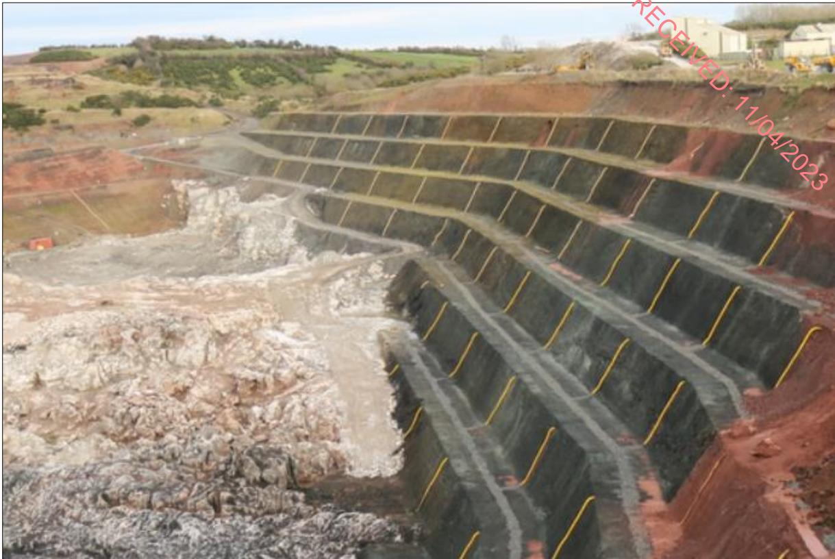
Figure 6: Drainage system of the pit slopes which will help reduce the contact of surface water runoff with gypsum materials once the level of the impounded water body rises
